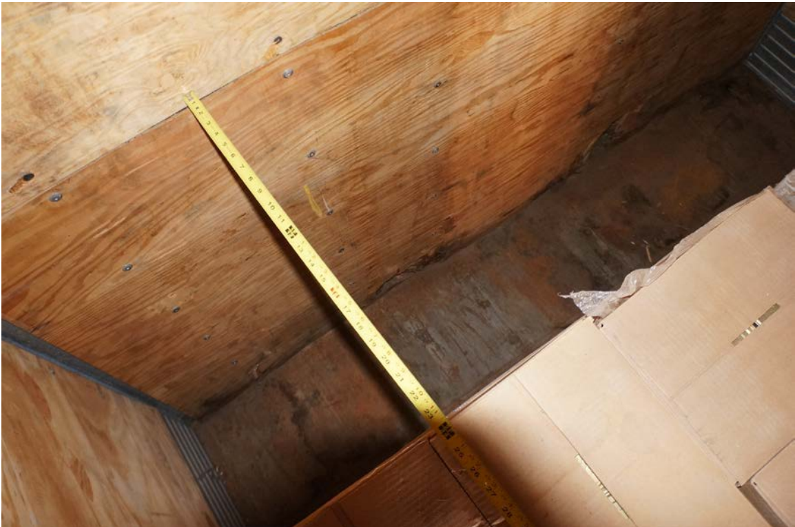
Longitudinal void space of 23 1/2 in. created after the 3 forward impacts
